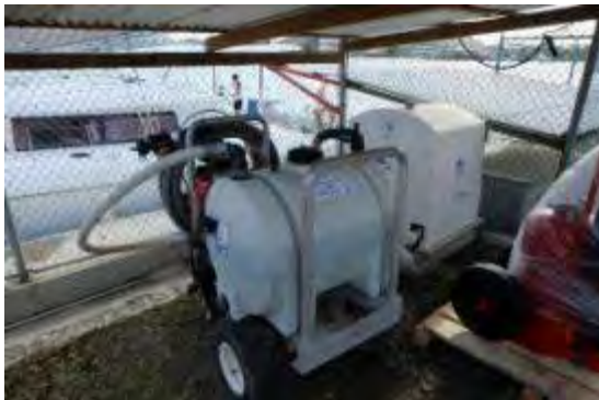
Picture 20: Mobile pump and onshore pumping station at IGY Rodney Bay Marina
