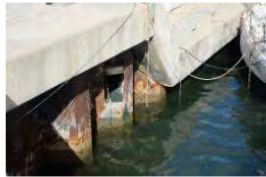
Picture 21: Effluent of the septic tank flowing into the Rodney Bay Marina
