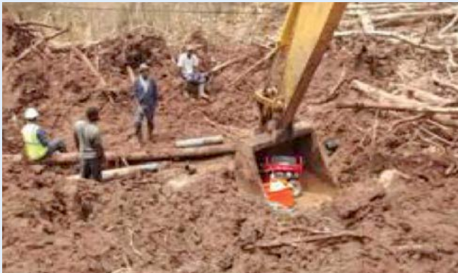
Dominica Water Infrastructure Post hurricane
